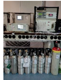
Fig. 2. Certification of Gas Mixtures Facility.
