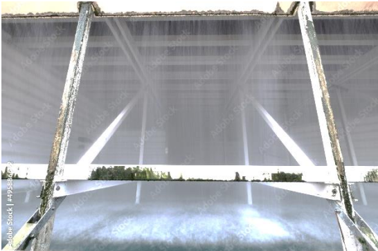
Biofilm in cooling tower
