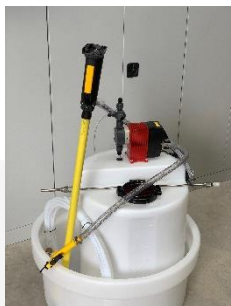
Chemical Dosing / Boiler feed tanksets
